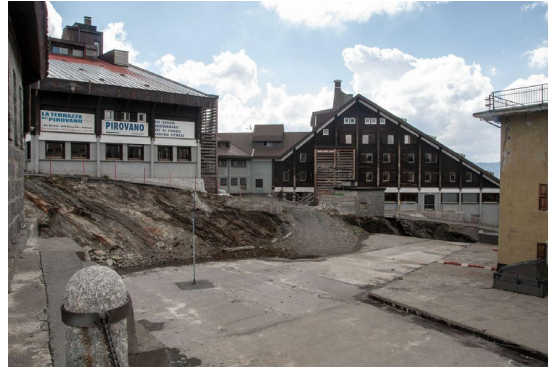
Figure 8: (a) Degraded public space at the top of Stelvio Pass. (b) Abandoned buildings of Casa Cantoniera IV
